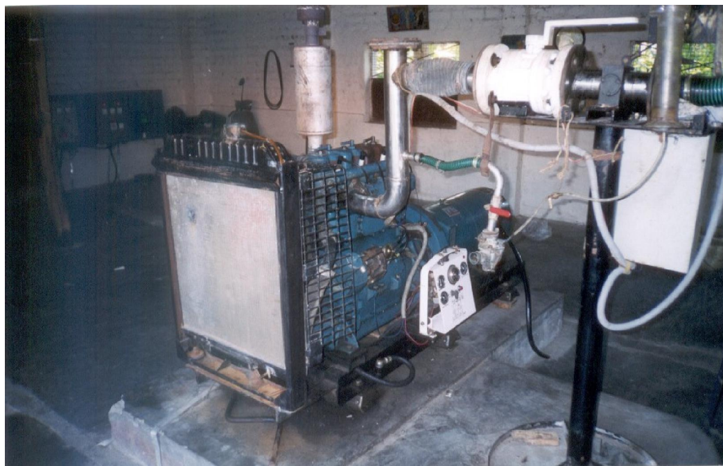
Plate 5.2 Producer gas engine at Dewan Estate, Bethmangala, Kolar District, Karnataka.
