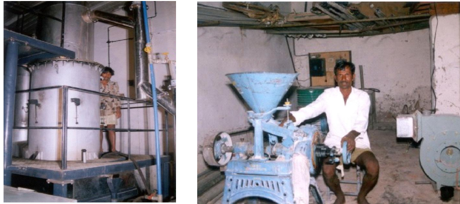
Gasifier Plant (Left) supporting Flour Milling Activity (Right) at Hosahalli
