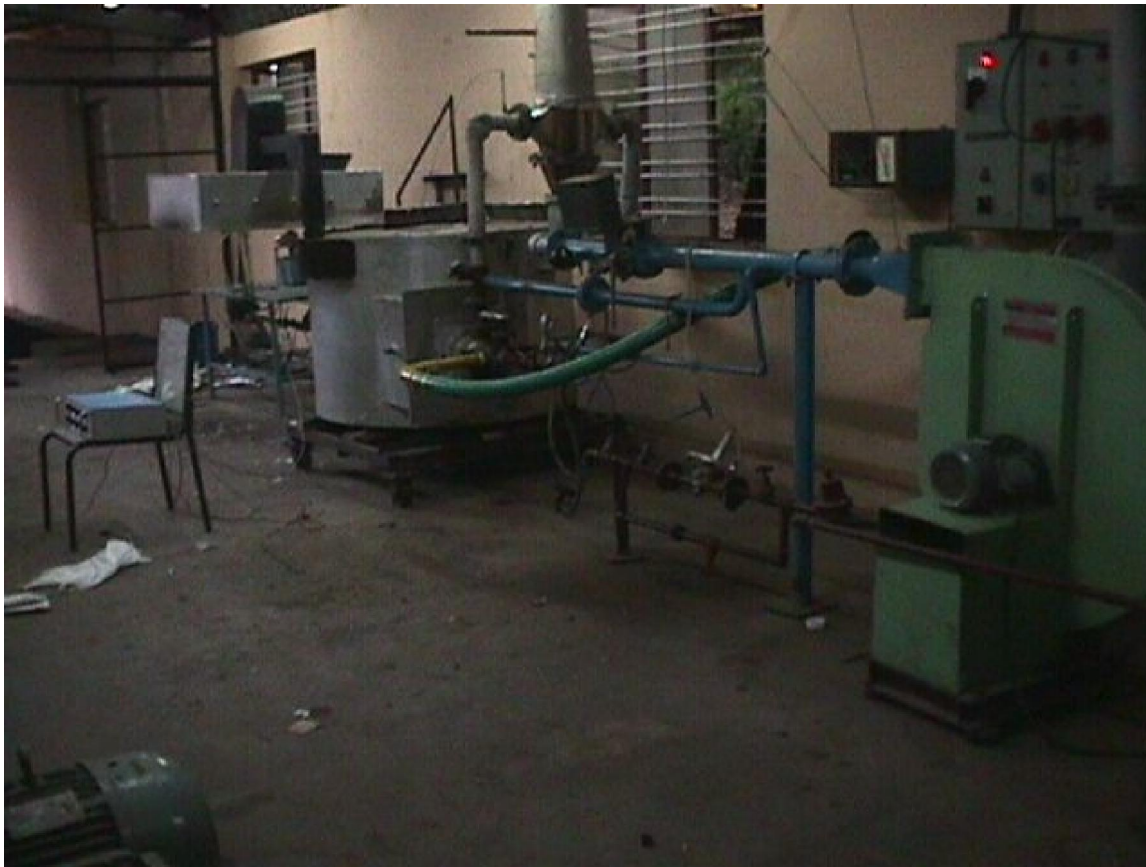
Plate 6.1 : The above photograph has a recuperator shown just below the top cone-like exhaust tubing. The air is forced from the blower through the recuperator and taken to the burner section of the furnace
